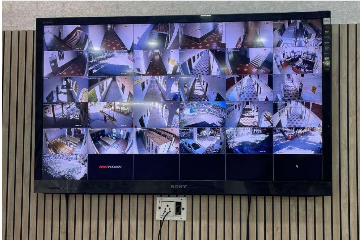
CCTV Surveillance in the Campus
